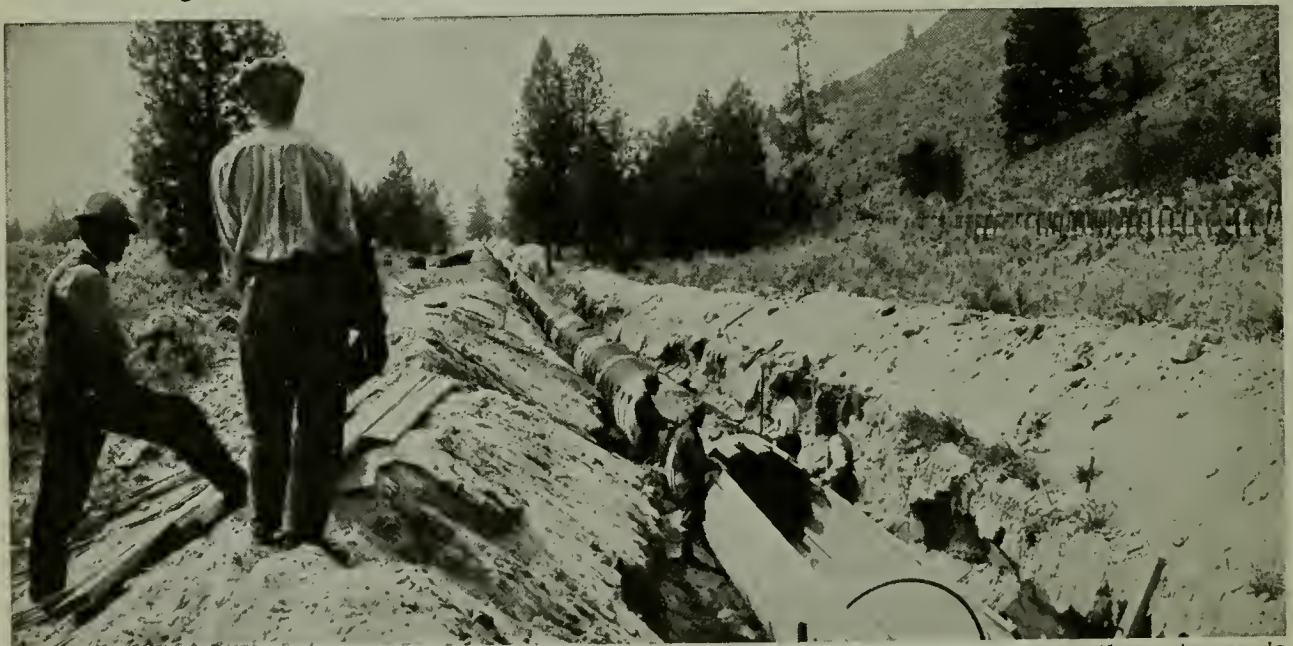
Where timber is plentiful wooden flumes, or pipes, are often laid in the trenches to carry the water, as is being done here in British Columbia. Iron rings inside and outside keep the planks in position.
